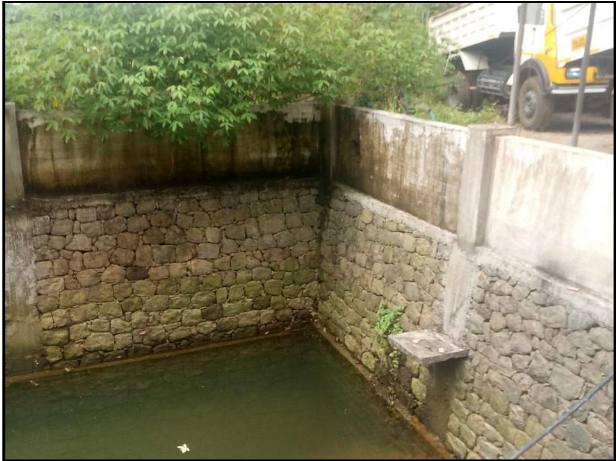
Photograph showing the rain water harvesting tank
